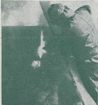
LIKE CUTTING CHEESE —the oxy-acetylene cutting blowpipe demolishes a 52-ton cast iron rock crusher bowl.
