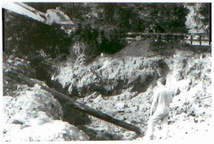
Fig. 4 Excavated telegraph pole at depth of four feet. Railroad bridge in background.
