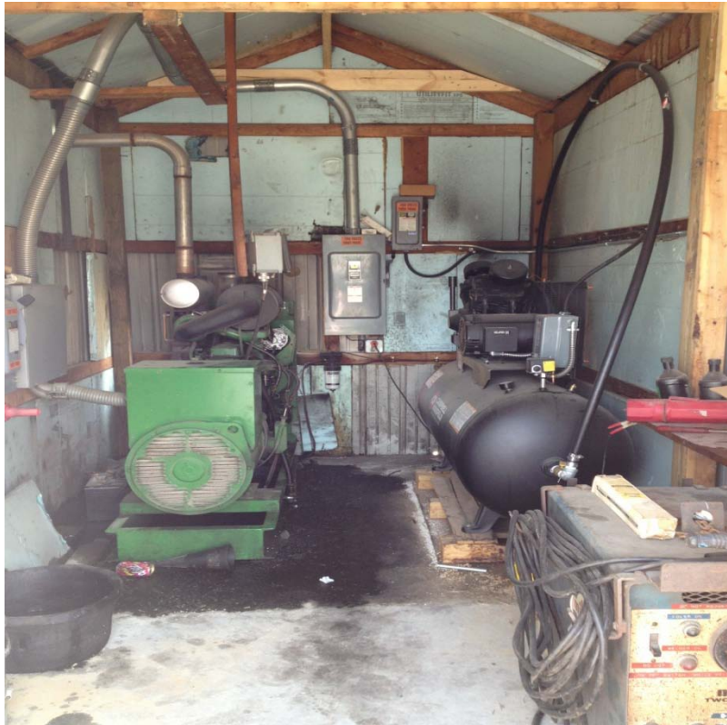
Figure 1: Industrial Diesel Generator
